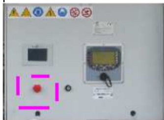
Emergency bottom on the control panel
